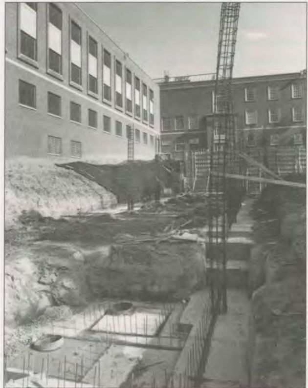
Construction of the Phase II expansion and renovation of the Law School building began last summer.
