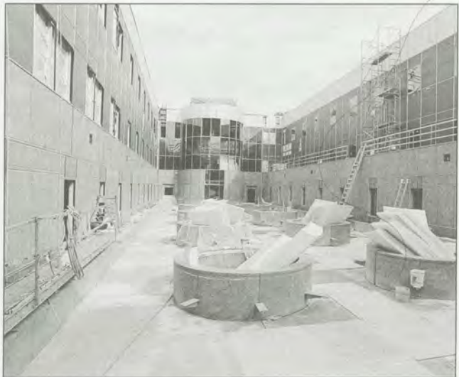
The courtyard between the existing building and the new addition nears completion.
